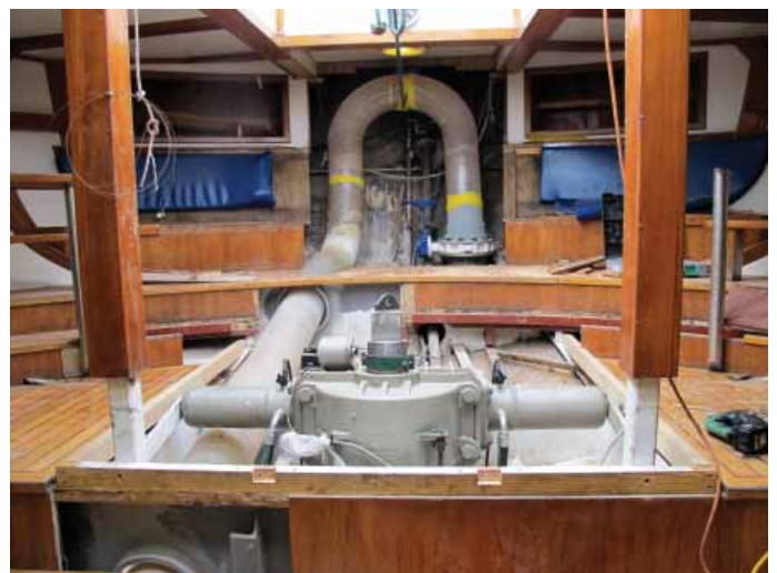
The new exhaust system sneaks past the rudder post and steering gear
